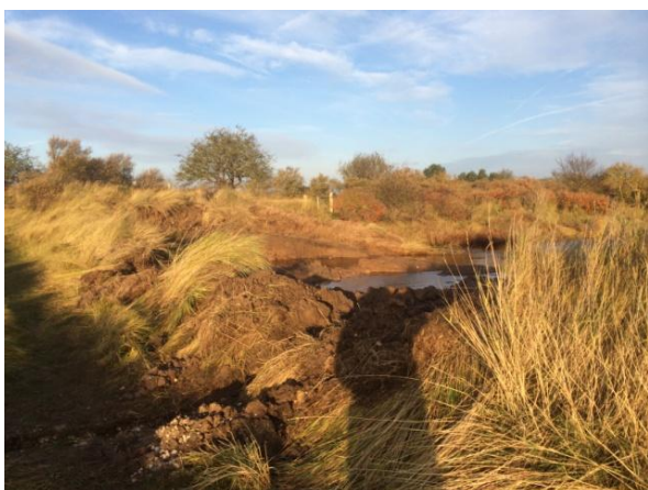
Breach point in Bulldog Bank Sluice
