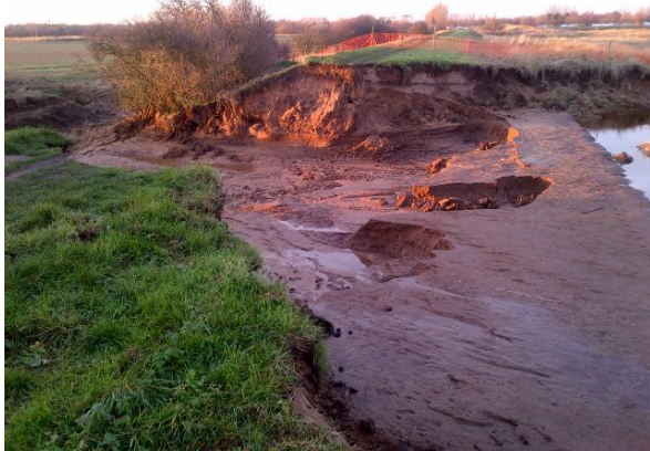
Breach on morning 06.12.13
