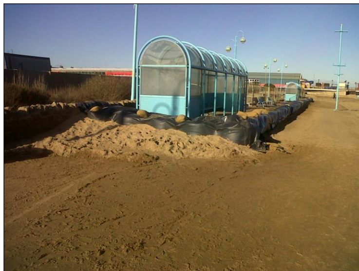
Damage to the flood wall
