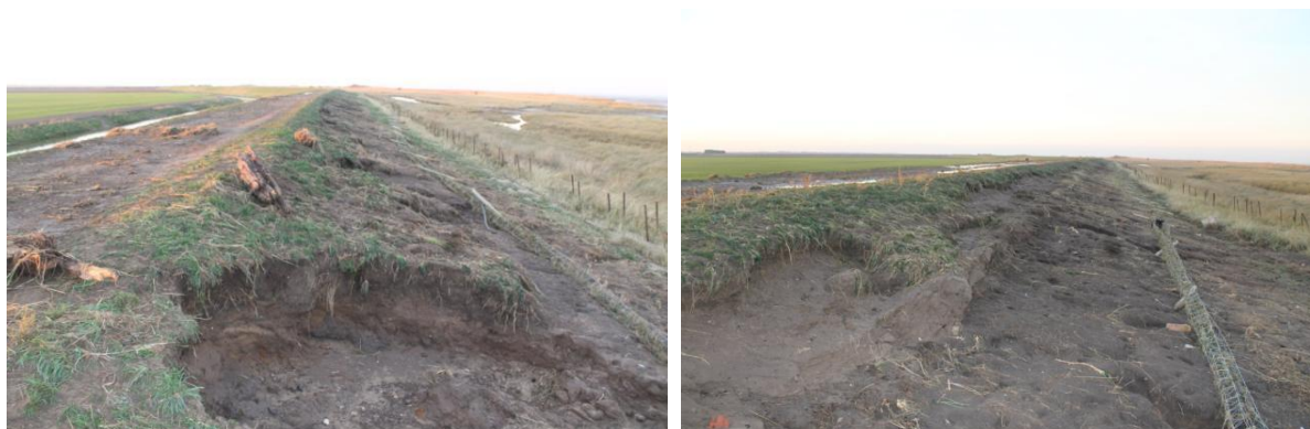
Damage to seaward face of embankment, primarily occurring up to the original crest level.
